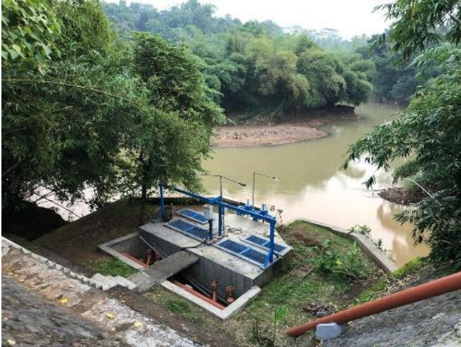
Intake Air Baku Sungai Ciliung
